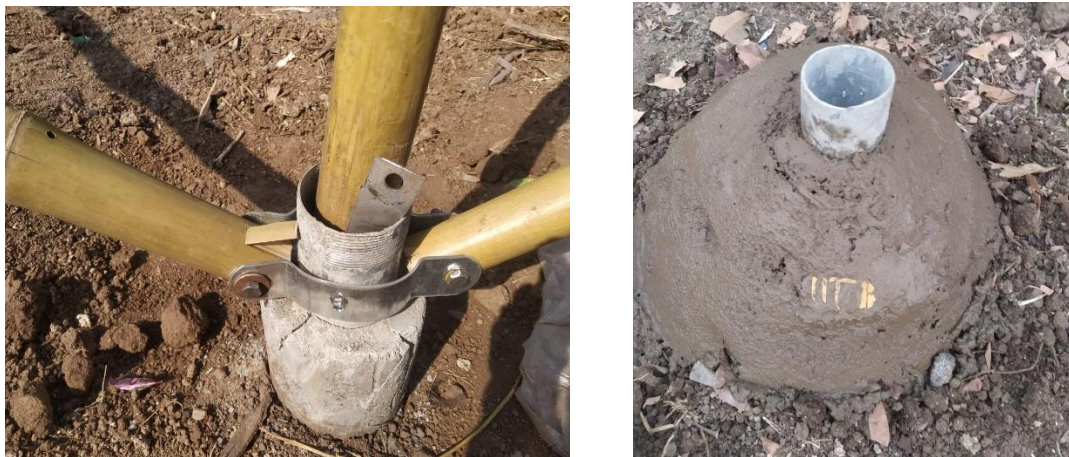
Figure 8. 3: On left – crack in Pre-Cast Foundation, On the right – in-situ foundation using cement mortar+sand+stones (Pictures captured at Balapur site)
