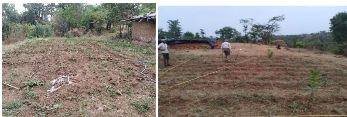
Figure 8. 1: Site selection and measurements made for the foundation for 1) on the left side- Balapur site 2) on the right side- Ramkhind site
