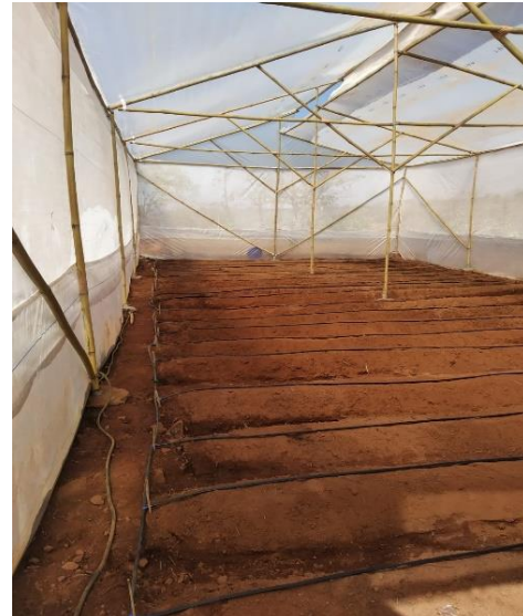
Figure 8. 14: Drip inlines place over the raised beds
